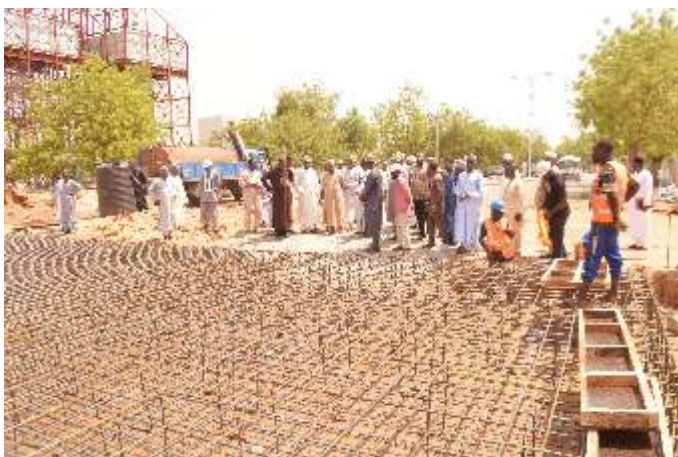
UMC led by VC, Prof. M. Y. Bello inspecting ongoing construction of BUK square
