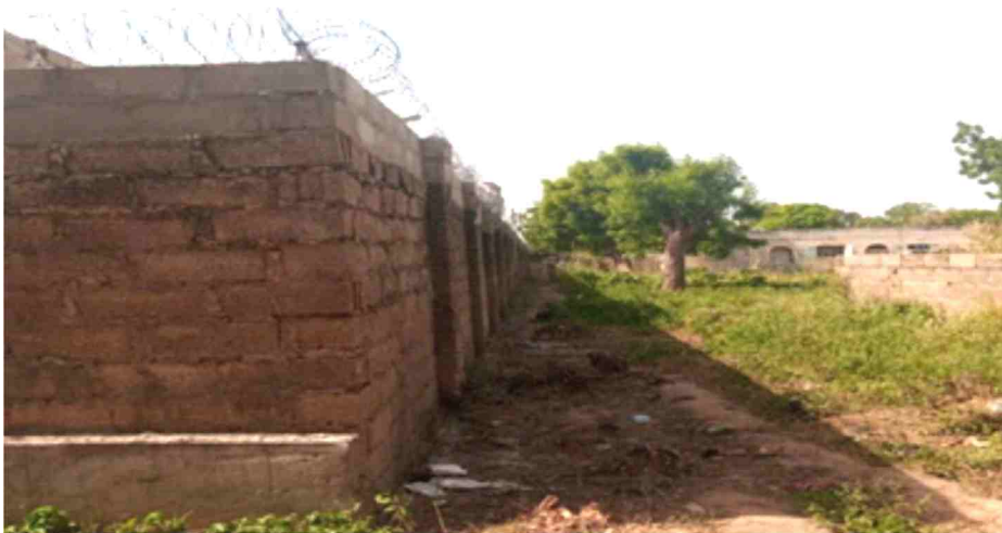
Construction of 1.5 high concrete wall and additional three coarse block wall at KUSUGU Crescent wall fence, Old Campus
