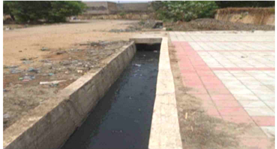
Drainage desalting at SCE
