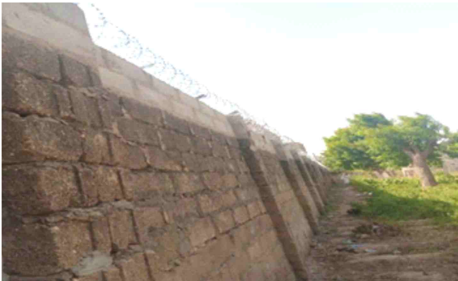
Increasing the wall height of the University fence at Old Campus along PAP-JAL Quarters, Yamadawa axis
