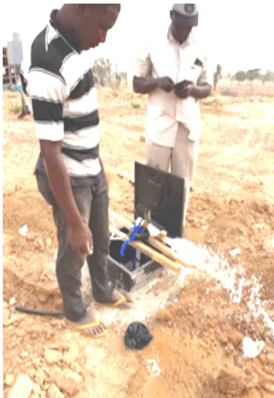
Construction of two nos. boreholes at tractor shed for Faculty of Law
