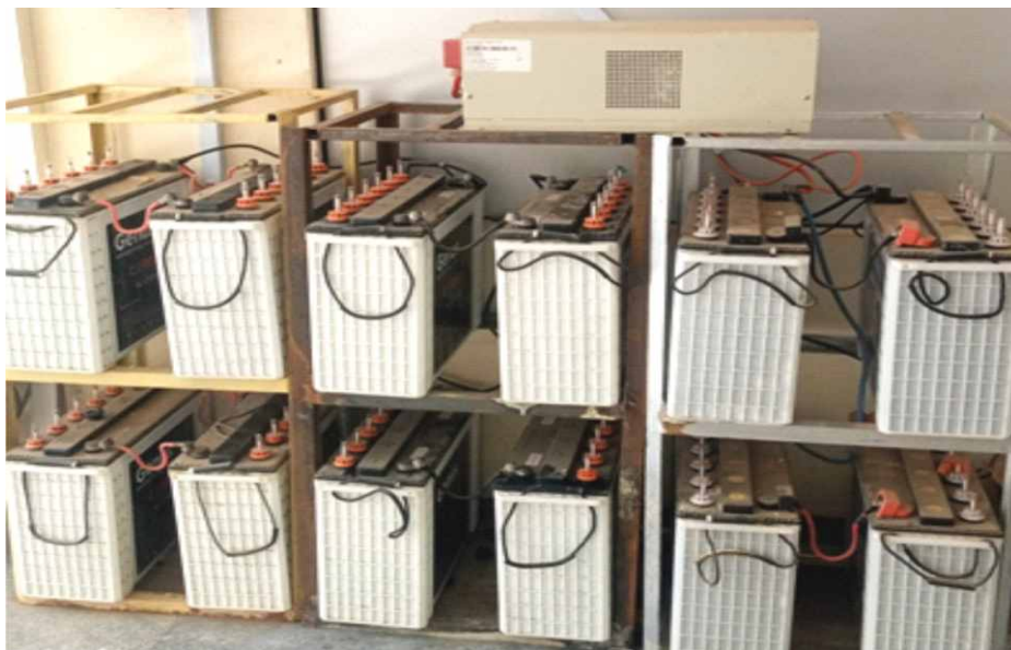
Figure 2 - 10KVA solar- inverter system
