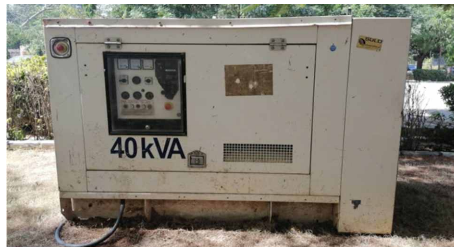
40 kVA Generator Purchased by the Research Groups
