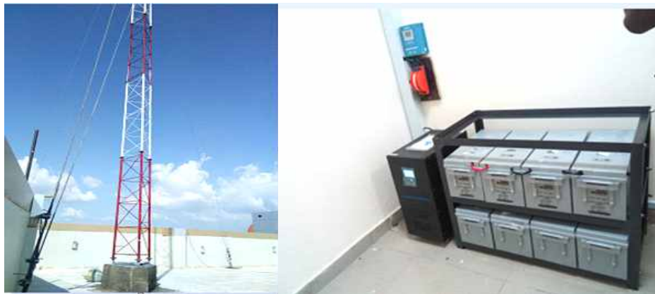
A Newly created network Mast and Eight Batteries bank donated by NCC (USPF) at Prof. Abubakar Rasheed Senate Building.
