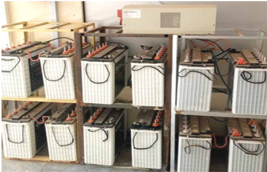
10KVA solar- inverter system
