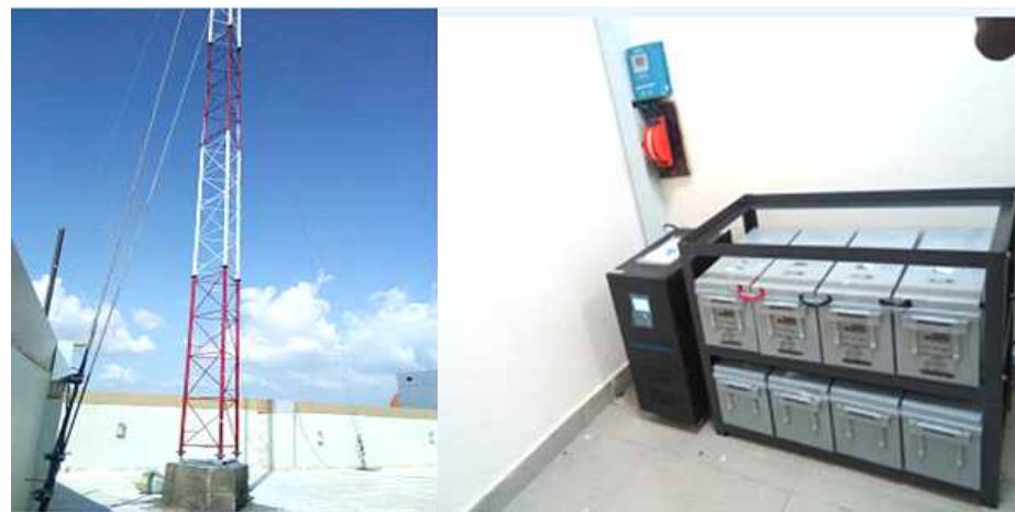
A Newly created network Mast and Eight Batteries bank donated by NCC (USPF) at Prof. Abubakar Rasheed Senate Building.
