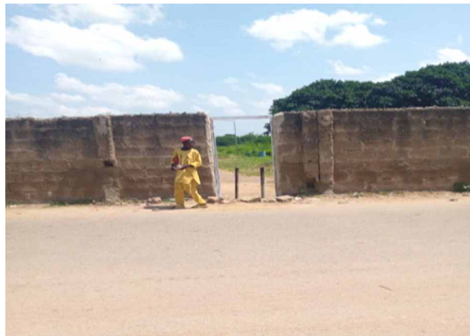
Repairs and provision of pedestrian gate at the Old Campus along the Yamadawa axis to ease linkages between the university and neighbouring communities
